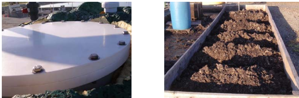
Figure 1. (A) Gas-tight hatch on east bioreactor; and (B) effluent drying and composting bin.
